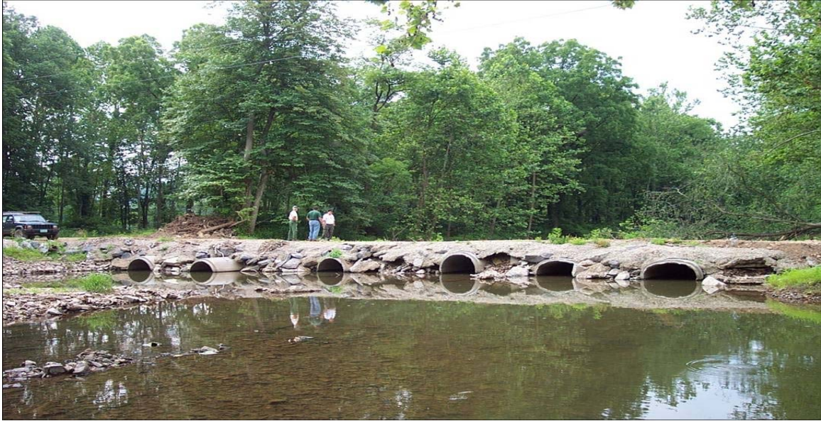
Photo 49. Water body is an RPW. This photo shows water flowing through a culvert. Culvert does not affect the jurisdictional status of the water body.
